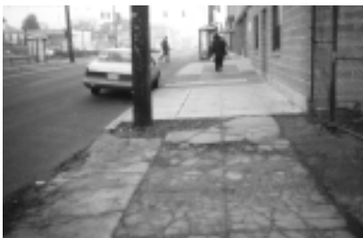
Some of the older sidewalk on Alberta Street is in disrepair.
